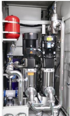
Fig. 4.23 Circulating Pure Water Cooling Cabinet
